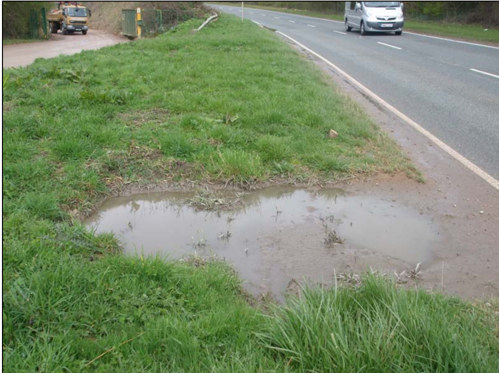
Photograph 1: Drainage issues at the entrance of Dunston Quarry B1188
